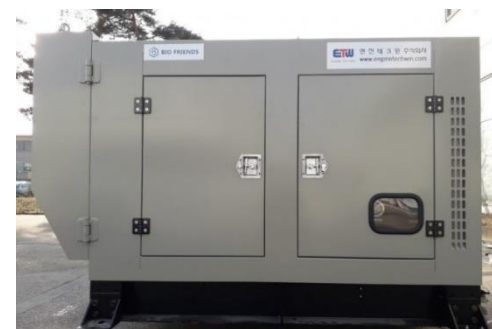
Bio Friends DME-fueled 40kW, 60hz generator developed with Engine Tech Win
