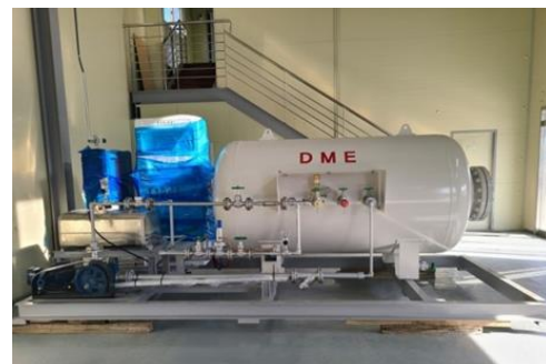
Bio Friends DME refueling skid - 3 ton capacity
